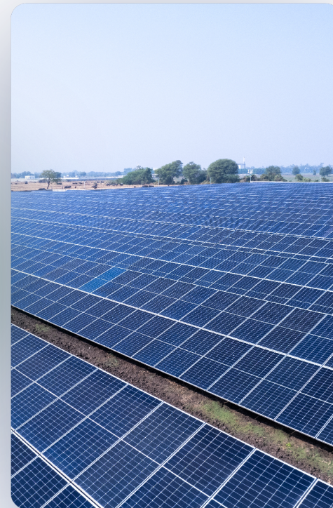
— ⚡ Utility scale generation
