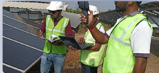
⚡ Live SCADA and drone thermography
